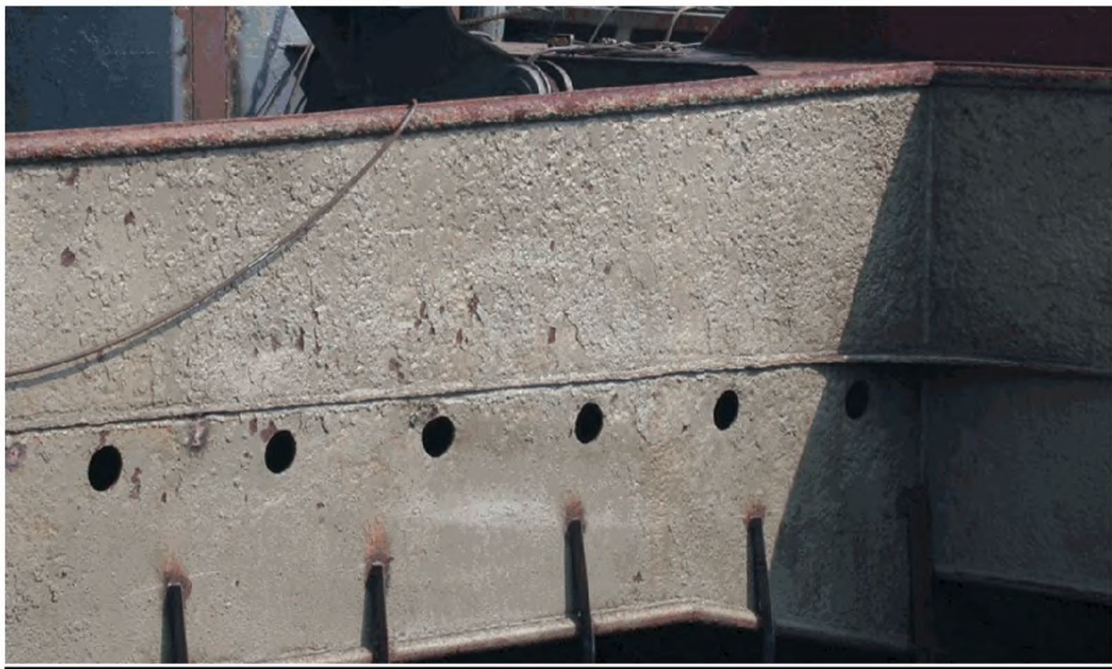
Photograph 1 Heavy corrosion of hatch coaming
