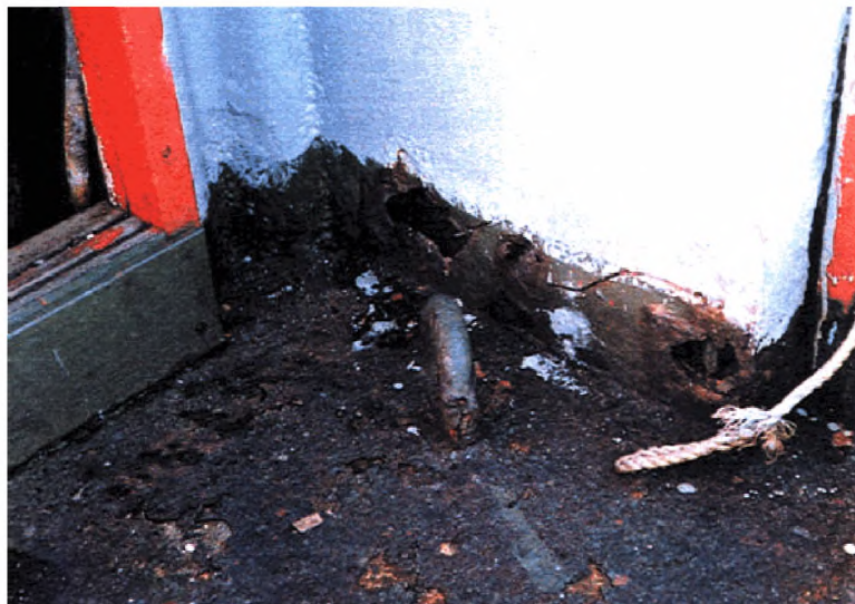
Photograph 1 Corroded accommodation house side structure
