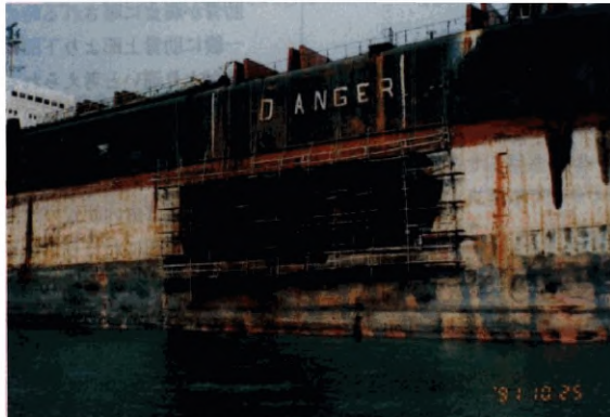
Photograph 2 Missing side shell structure (See Examples 4 and 5)
