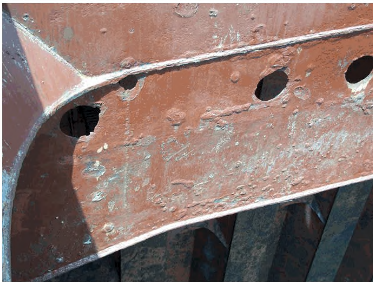
Photograph 2 Heavy corrosion of hatch coaming
