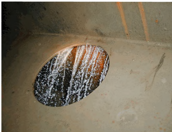
Photograph 1 Side shell fracture in way of horizontal stringer weld
