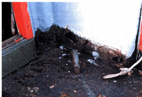
Photograph 1 Corroded accommodation house side structure
