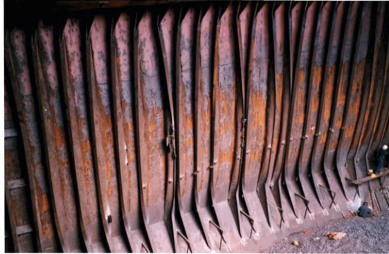
Photograph 1 Collapsed side shell frames (See Example 4)
