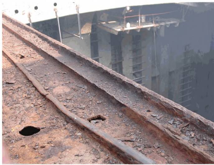
Photograph 4 Corrosion at the top of the hatch coaming
