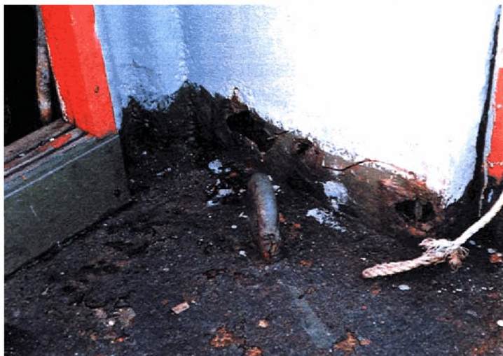
Photograph 1 Corroded accommodation house structure
