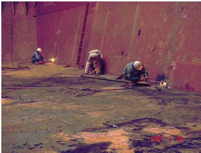
Photograph 1 Heavy corrosion affecting inner bottom plating
