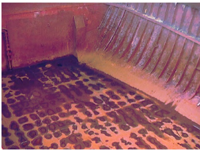
Photograph 2 Damaged inner bottom plating
