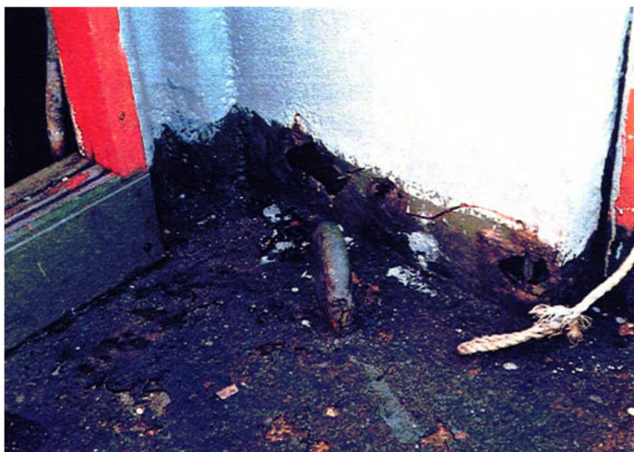
Photograph 1 Corroded accommodation house structure
