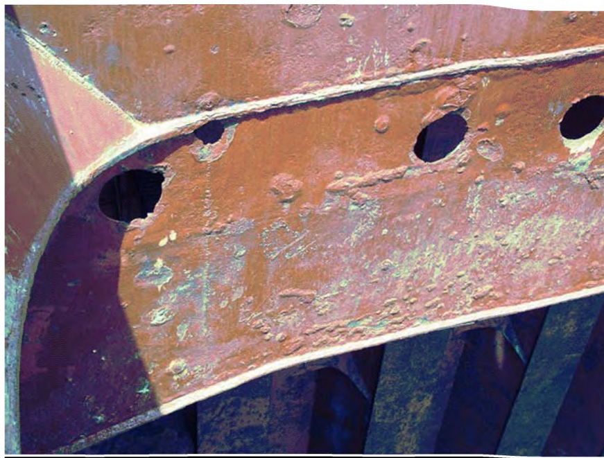
Photograph 2 Heavy corrosion of hatch coaming
