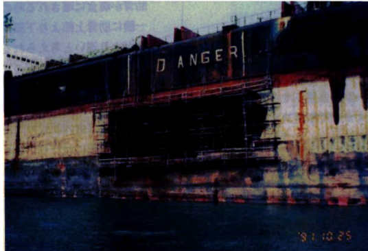
Photograph 2 Missing side shell structure (See Examples 4 and 5)
