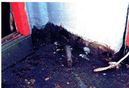
Photograph 1 Corroded accommodation house side structure
