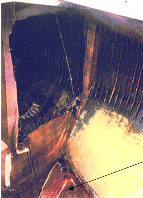
Photograph 1 Collapsed and detached transverse bulkhead
