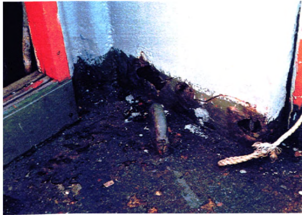
Photograph 1 Corroded accommodation house structure
