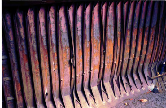
Photograph 1 Collapsed side shell frames (See Example 4)
