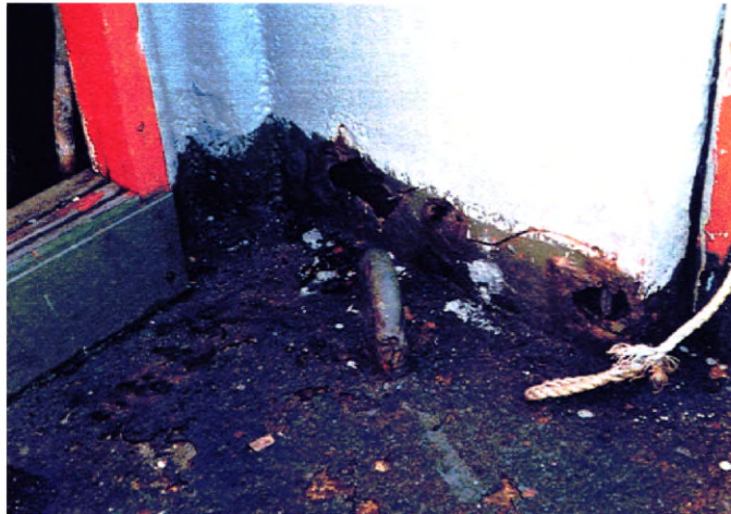
Photograph 1 Corroded accommodation house side structure
