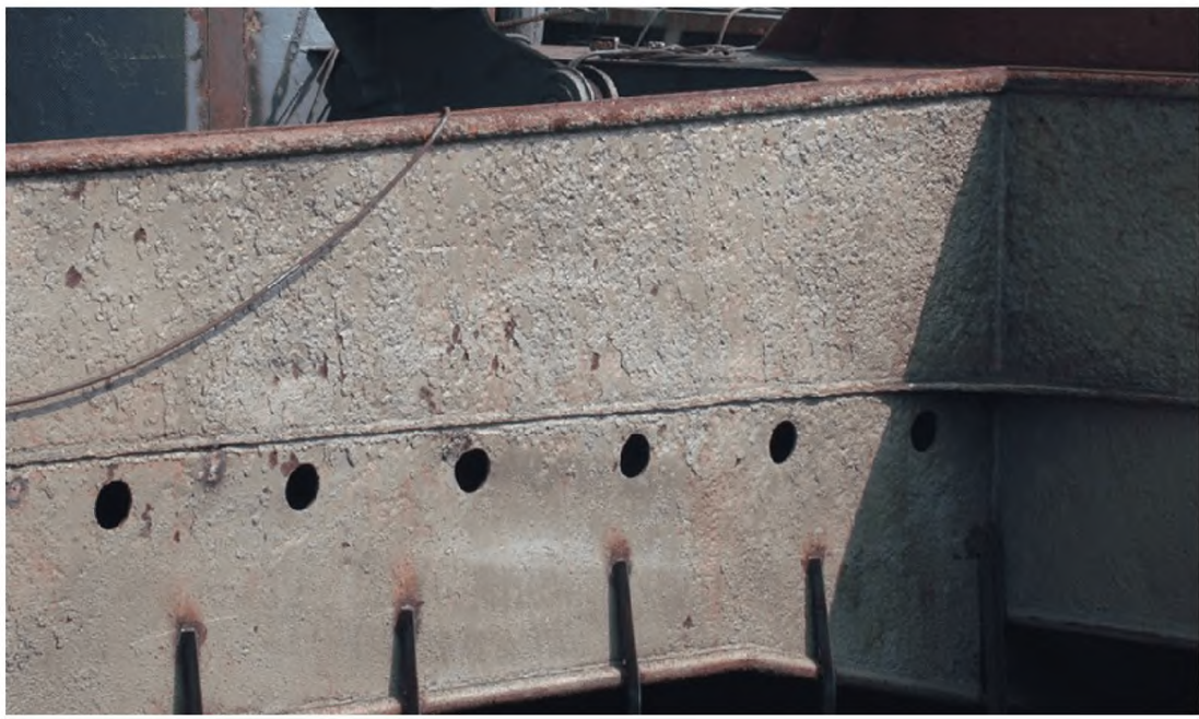
Photograph 1 Heavy corrosion of hatch coaming
