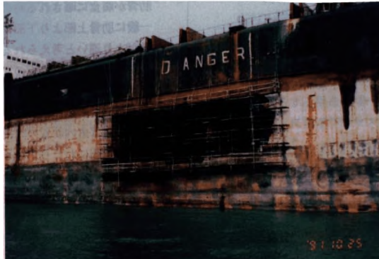
Photograph 2 Missing side shell structure (See Examples 4 and 5)
