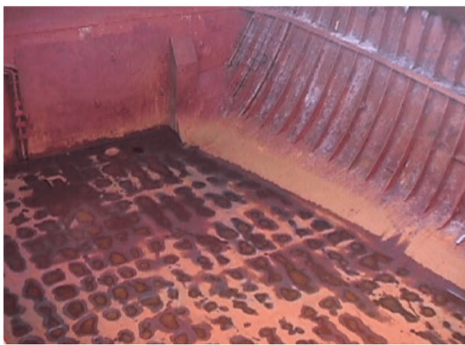
Photograph 2 Damaged inner bottom plating
