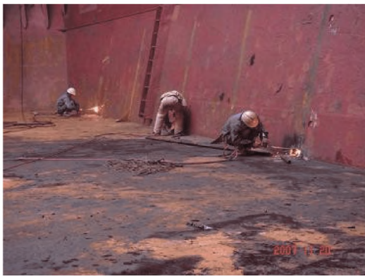
Photograph 1 Heavy corrosion affecting inner bottom plating
