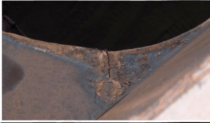
Photograph 3 Fractures at the hatch corner
