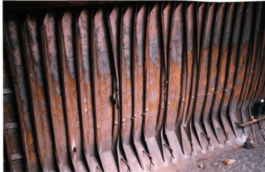
Photograph 1 Collapsed side shell frames (See Example 4)
