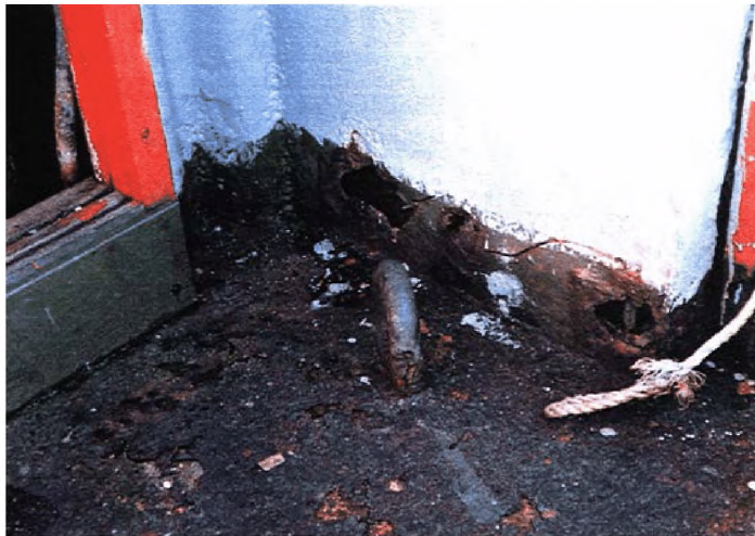
Photograph 1 Corroded accommodation house structure
