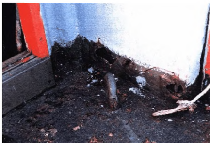
Photograph 1 Corroded accommodation house side structure
