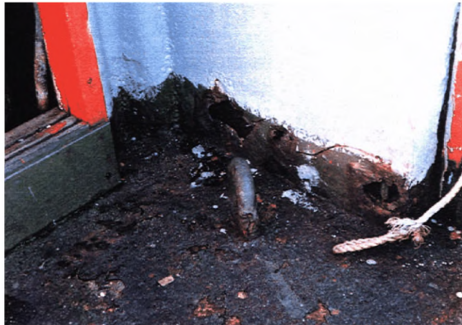
Photograph 1 Corroded accommodation house side structure
