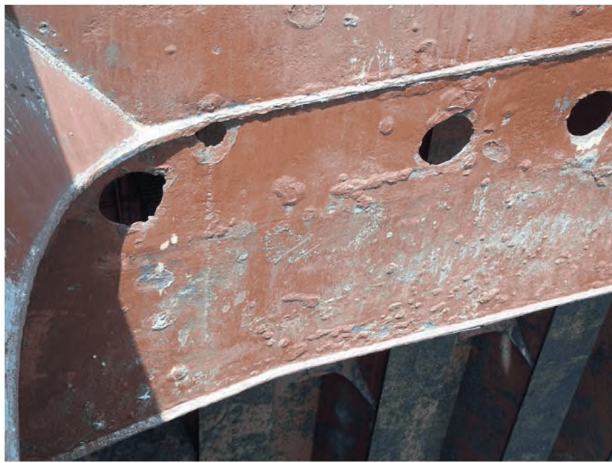
Photograph 2 Heavy corrosion of hatch coaming
