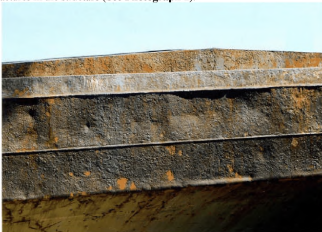
Photograph 1 Heavy corrosion of hatch coaming and topside tank plating vertical strake
