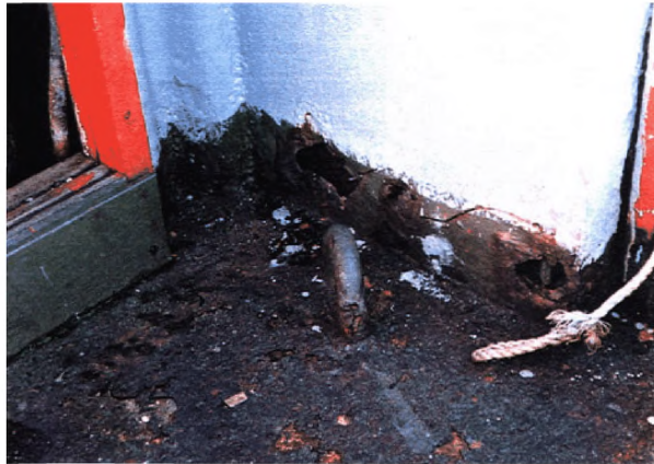
Photograph 1 Corroded accommodation house structure
