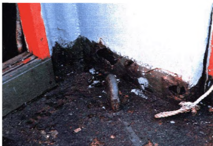
Photograph 1 Corroded accommodation house side structure
